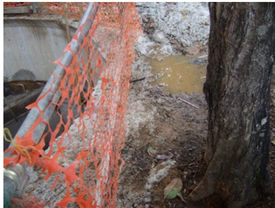
Figure 5: Construction cement deposited at tree base.
