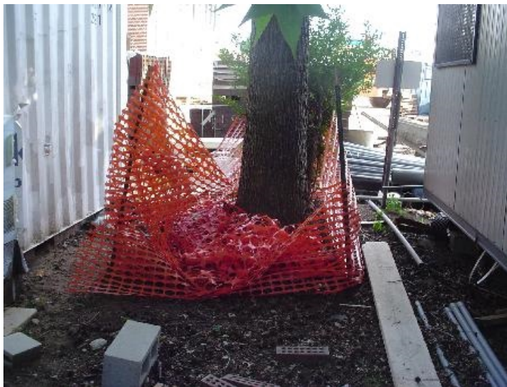
Figure 7: Inappropriate installation/maintenance of TPZ during construction.
